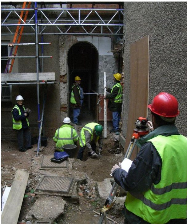
Above: EAS members in full safety gear working in Forty Hall courtyard in May, as part of the renovation work. (Photo: Editor)
